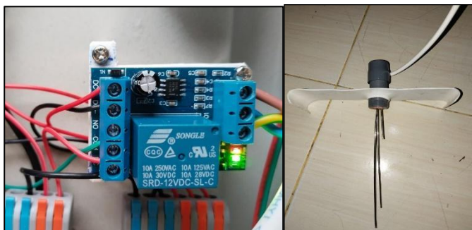
Gambar 5.7 Implementasi Liquid Level Controller Sensor
